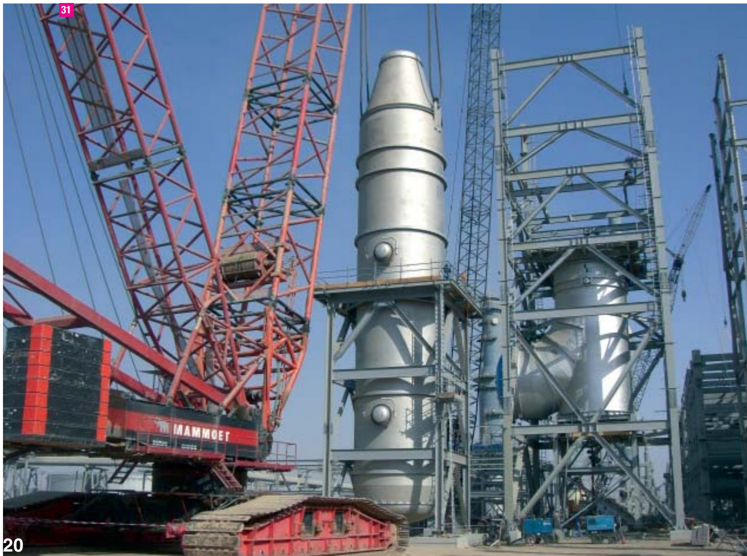
31 Orifice Chamber, CS w/ refractory lining, JGC Co. - ARAMCO, Rabigh refinery, Saudi Arabia
