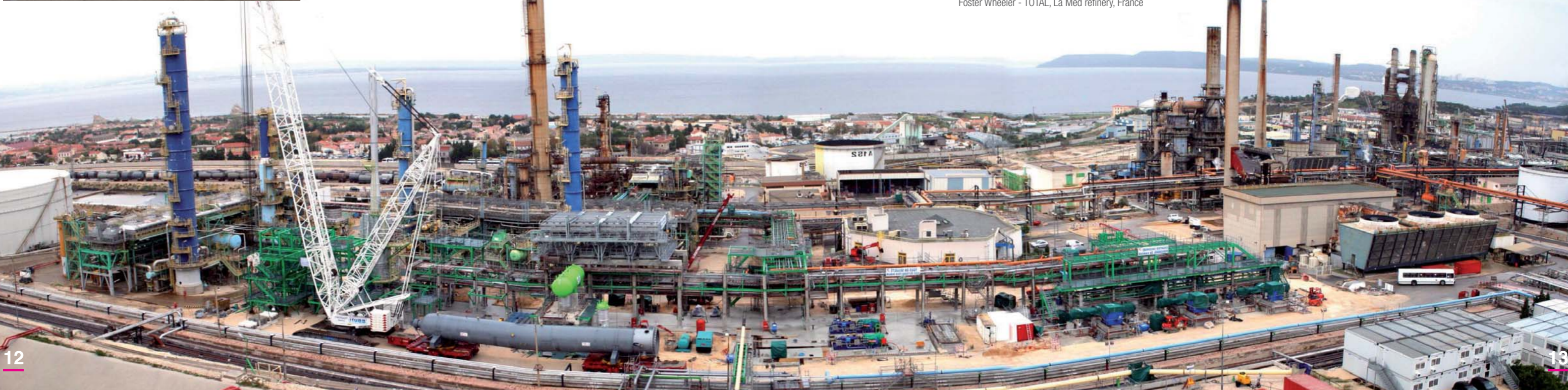
11 HDS Reactor (350 ton), 2.25 Cr alloy w/ 347 SS.W.O., Foster Wheeler - TOTAL, La Med refinery, France
